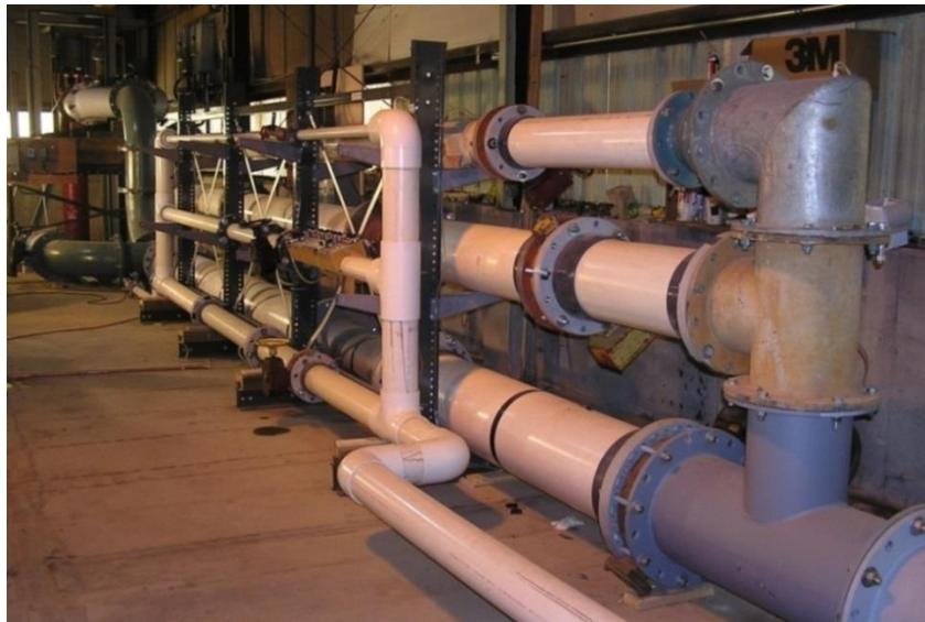
Figure 4: Photograph Showing Laboratory Flow Meters
