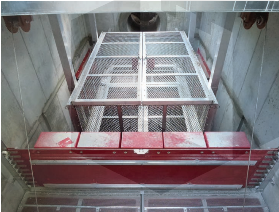
View of Nutrient Separating Baffle Box and SkimBoss Upflow Filter
