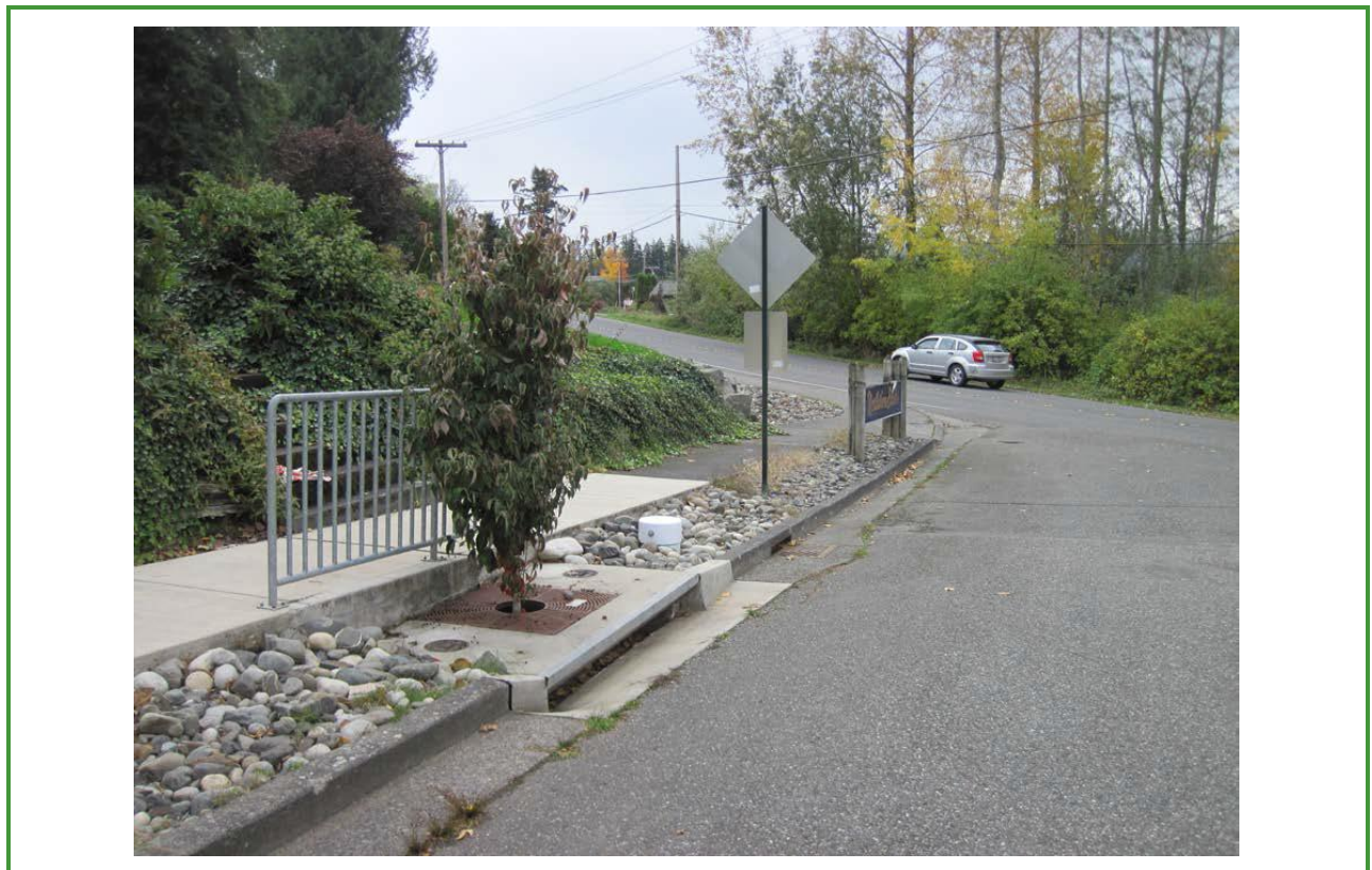
Figure 3. Photograph of the Filterra System on Hayward Drive.
