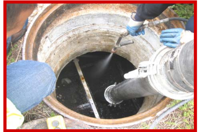
Insert Vacuum Hose in the Sedimentation Chamber and Vacuum Out All Trash, Sediment and Standing Water.
