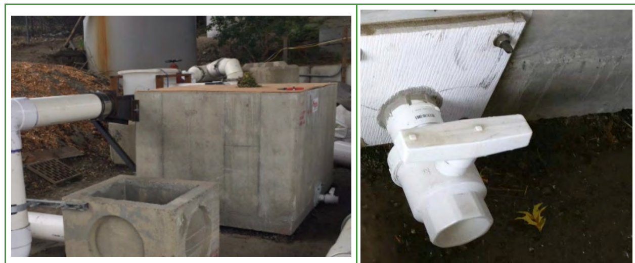
Figure 2. Photos of StormGarden Test System with Filter Panel Valve on the Right Bottom Wall.
